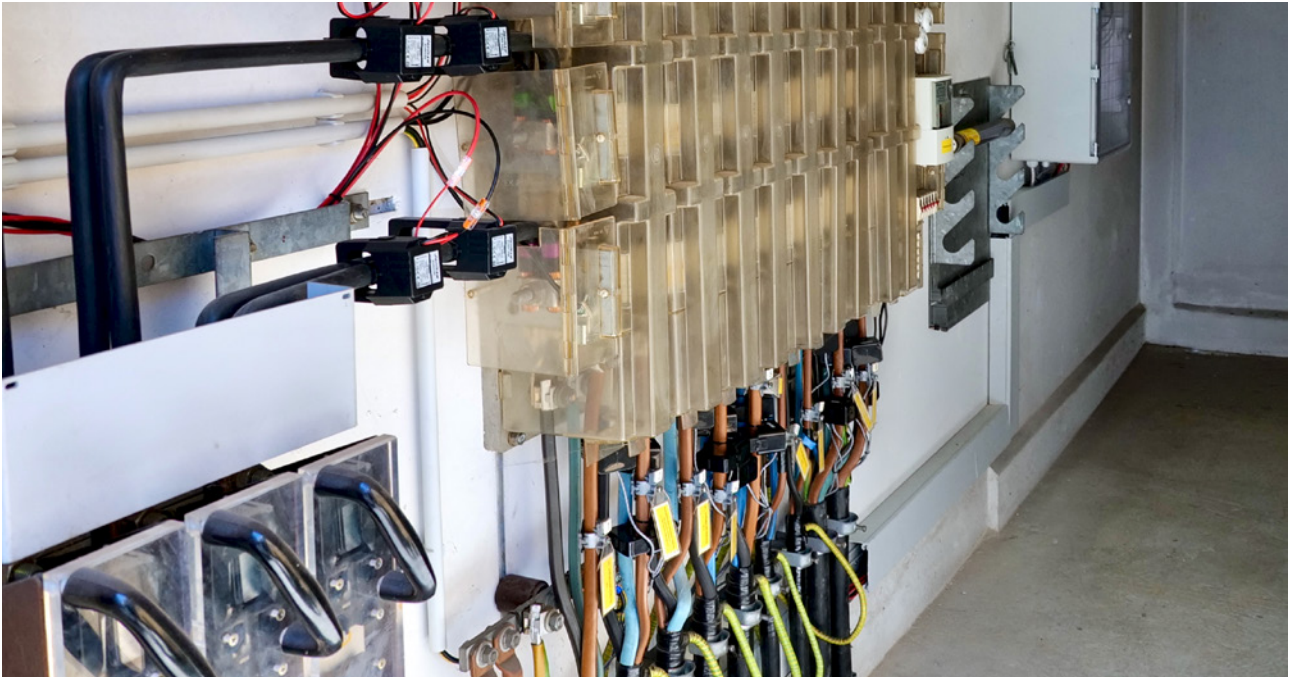
Even older local distribution substations dating from the 1980s can be digitalized using Janitza measurement technology
