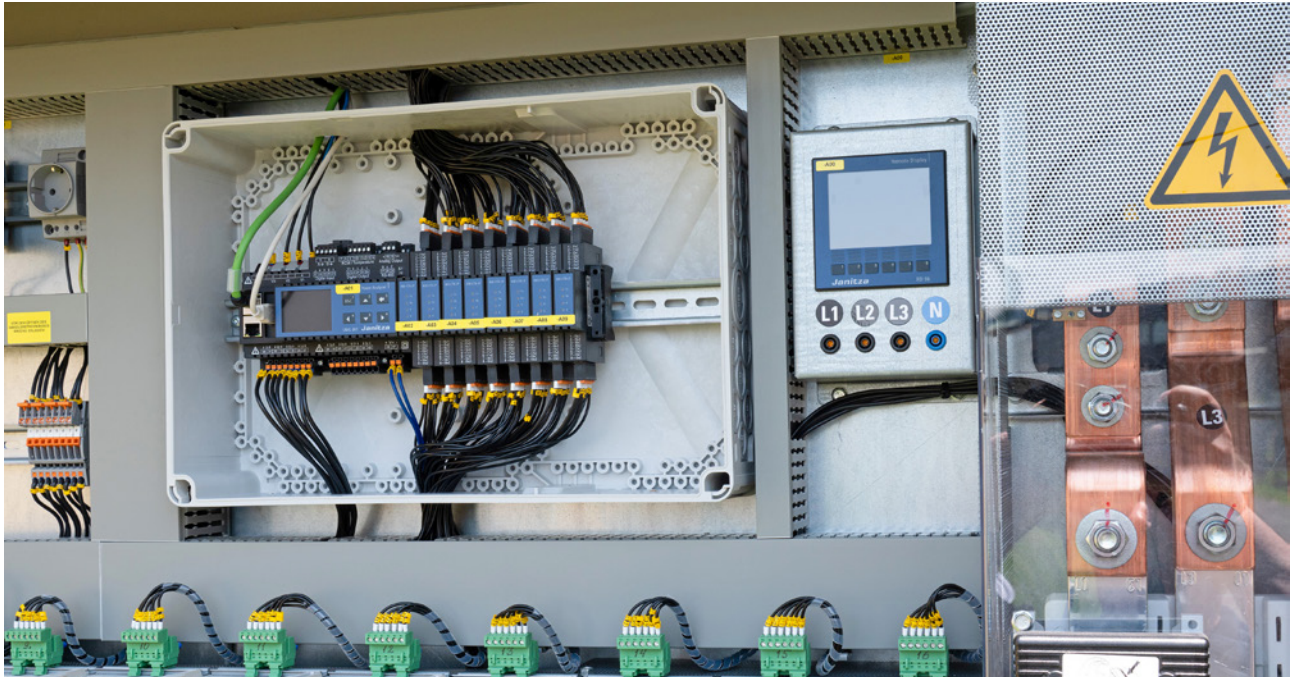
Space-saving: expandable modular power analyzer UMG 801 with 800-CT8-LP current measuring modules and Remote Display RD 96 in a new station
